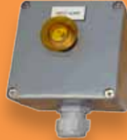
reset unit in wall box pre-alarm indication bridge & open bridge wings WAR 220.2.0.0
